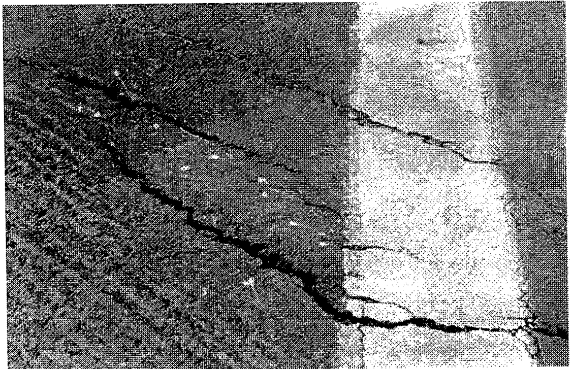
Figure 7. Cracking in the Areas of Heaving (SH 161)
