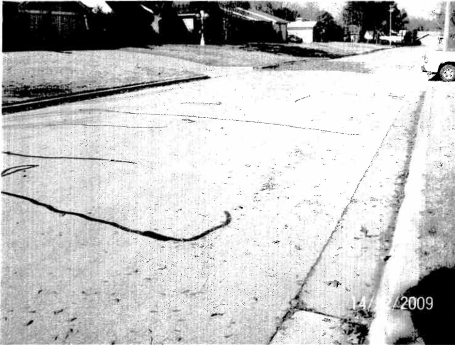
Picture #3-Untreated area-Note extensive shrinkage cracking. No trees in this area.
