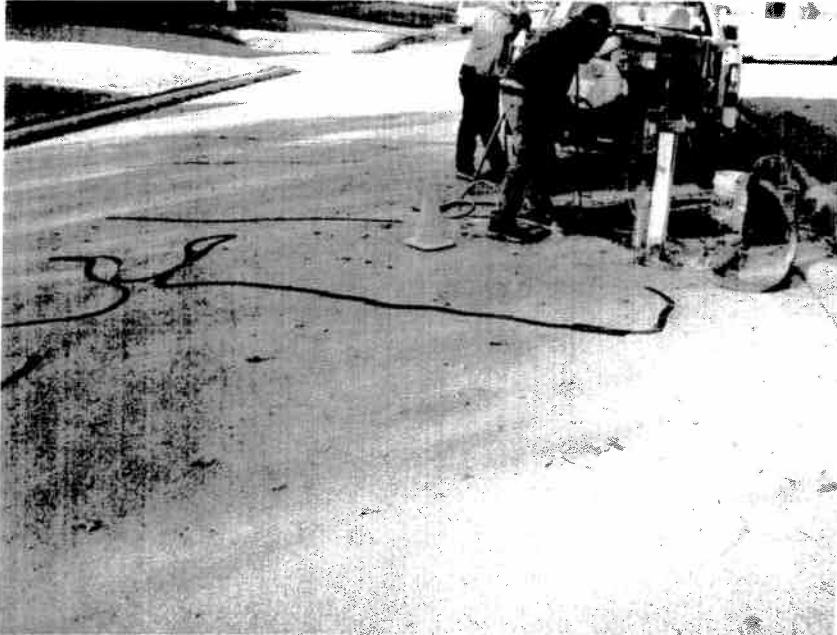
Picture #2-Sample taken from untreated area-recently crack sealed with asphalt.
